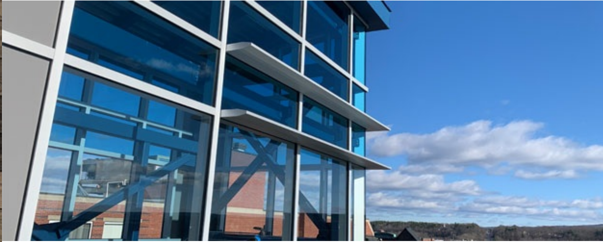
Photo: New five-story stair tower for renovated parking garage, to be featured in the Spring Newsletter
